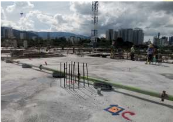
Figure 10b Data acquisition for the points height level of points in the study area is conducted using a levelling instrument for monitoring purposes
