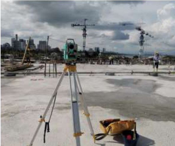
Figure 10a Data acquisition for the X, Y coordinate locations in the study area is conducted using a Total Station for monitoring purposes
